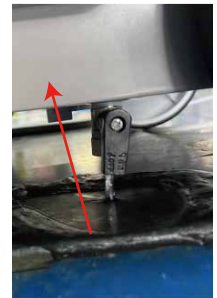
Drainage valve open
